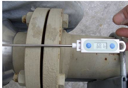
Initial Reading prior to coating of Industrial Insulation Coating reading 75.2°C and 68.1°C on picture to the right.
